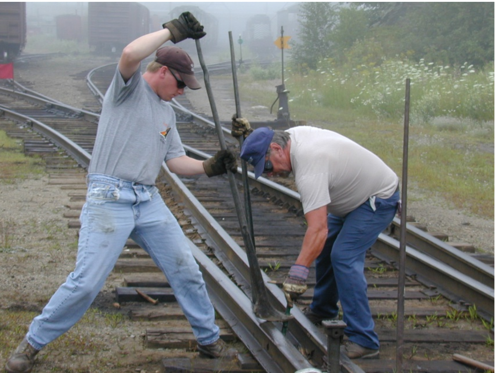
On July 31, 2000, Rod photographed this pair, Don Hogan on the right, working on the track outside the locomotive servicing facility at NMJ. Rod Bushway photo
