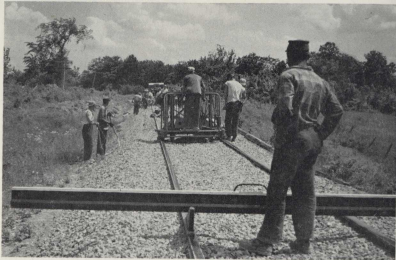
After ballast is spread on clean roadbed, and before tamper passes over new ballast, a crew uses a spot board (foreground) and power jack to assure maintenance of grade.
