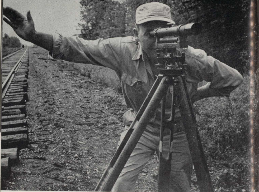
Brief Aroostook summer finds BAR track maintenance crews taking advantage of warm weather for major track repair. Above, Clayton McCue, behind level, signals partner along a stretch of problem track.
