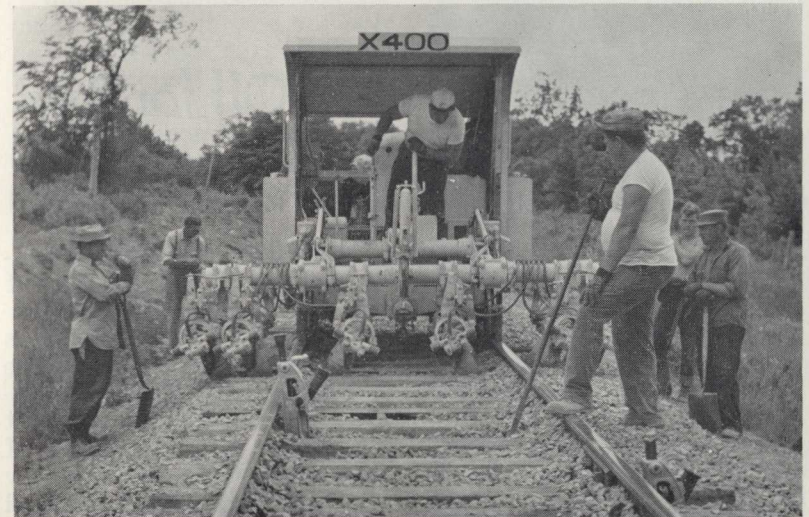
Final operation in cleaning and reballasting is tamping crushed rock ballast firmly around ties. Multiple tamper, pictured below, eliminates nearly all hand tamping. Hydraulically-controlled steel fingers do the job.
