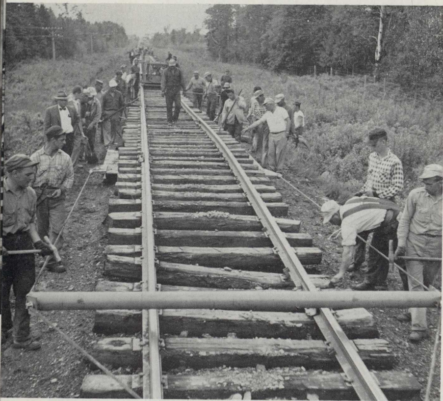
Diesel Units in tandem furnish power for plow. Crew follows, removing defective ties, inserting new ties and relining track.
