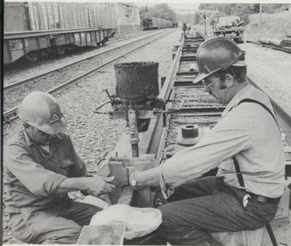
Mayberry and Section Foreman Paul Michaud (left) prepare a sand mold which will hold a mixture of iron oxide and aluminum that's fired to produce welding heat. The thermit weld is normally a procedure that's confined to field use but the amount of rail to be welded was not large enough to bring in a contract welding operation.
