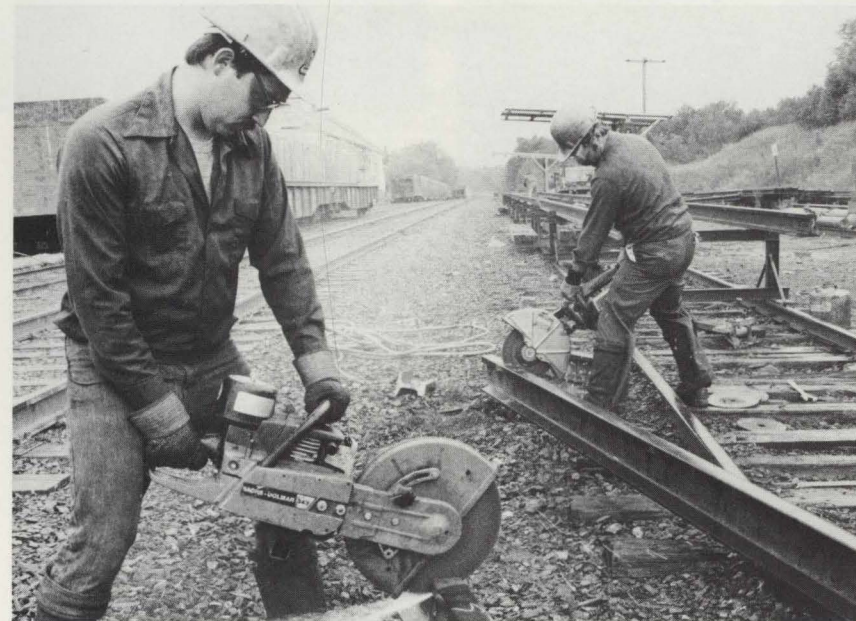
Wayne Lunn (left) and Lomen Fournier use rail saws to crop the ends of relay rail prior to the welding. Extra holes are drilled in the welded 76-foot rail so that six-hole joint bars can be used when the rail is laid. The result is steel that's nearly as strong as the "ribbon rail" which BAR has installed.
