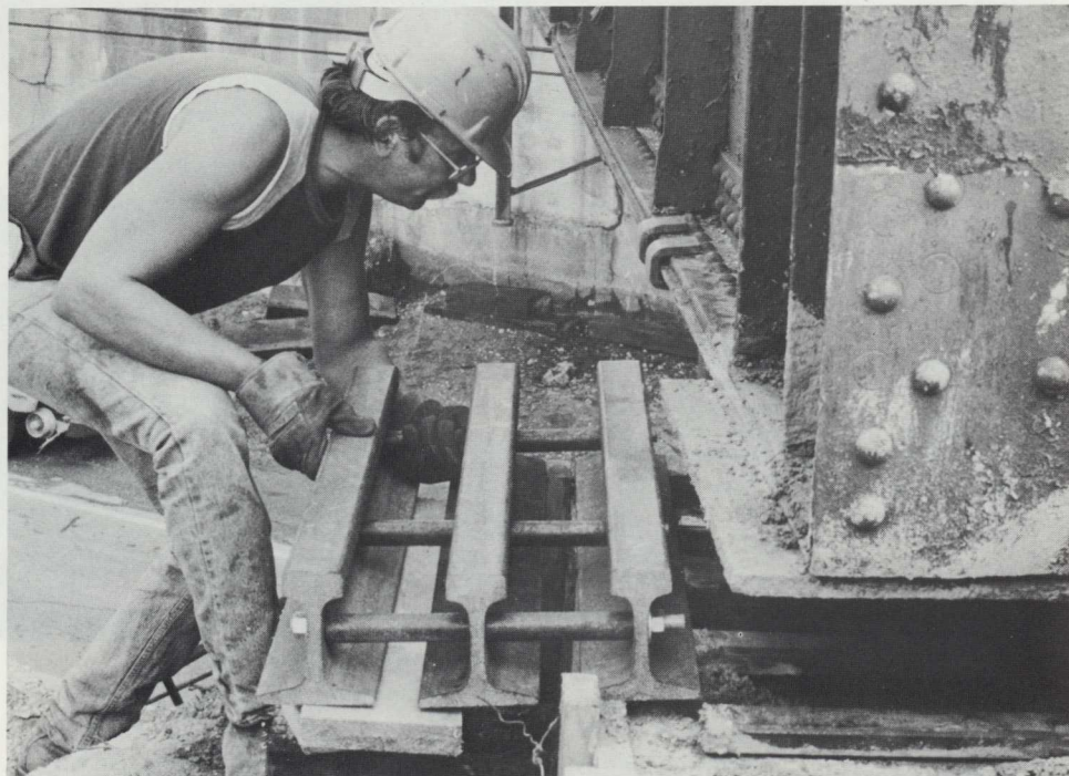
Fred Thayer fits a grillage — steel rail that's been cut and welded into cubes — under the bridge. The grillage will eventually be encased in concrete and serve as a part of a new bridge support.
