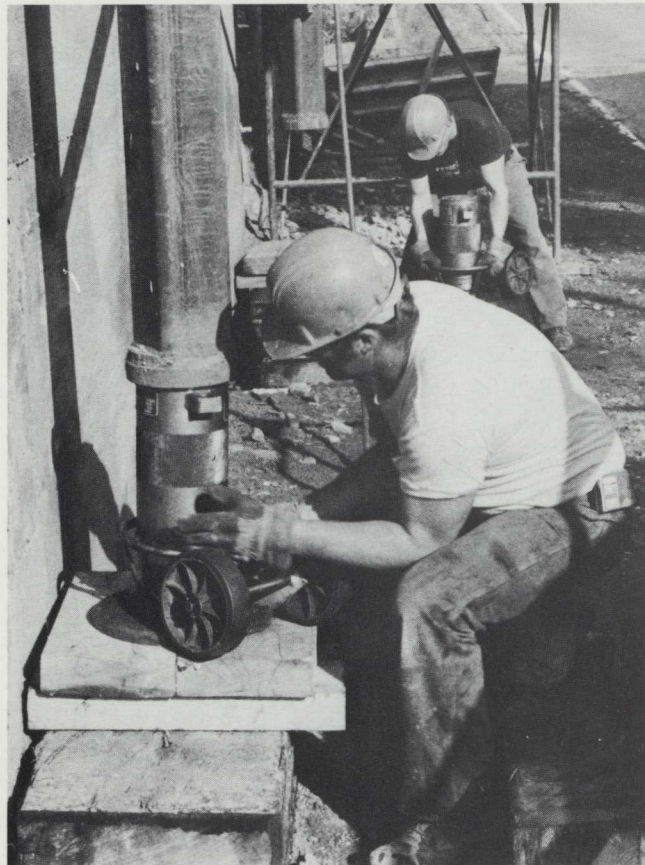
Fred Brawn places one of the heavy duty car jacks under the jacking frame prior to a lift.
