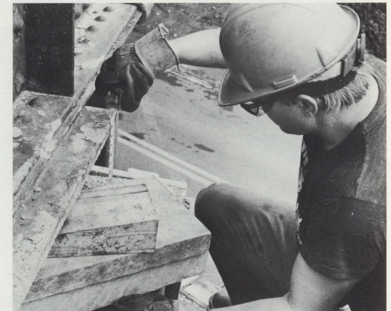
The frame permitted the use of longer jacks than would otherwise have been possible, enabling crews to raise the bridge in six-inch lifts. Carpenter Bob Thibodeau takes a measurement while the crew on the ground control the jacks.
