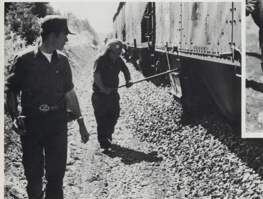
Acting Roadmaster Bob Huston pitches in as the Ballast Crew dumps new rock north of Portage.
