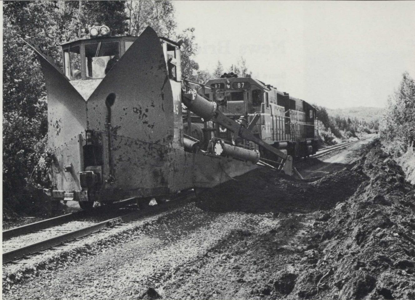
Superintendent of Track Brian Baker got a deal he couldn't refuse this year: all the rock ballast his people could install. As a result, BAR will install more rock ballast this year than any time since the construction, about 95,000 tons. Jordan spreader cleans the shoulders of the track prior to the installation of ballast.
