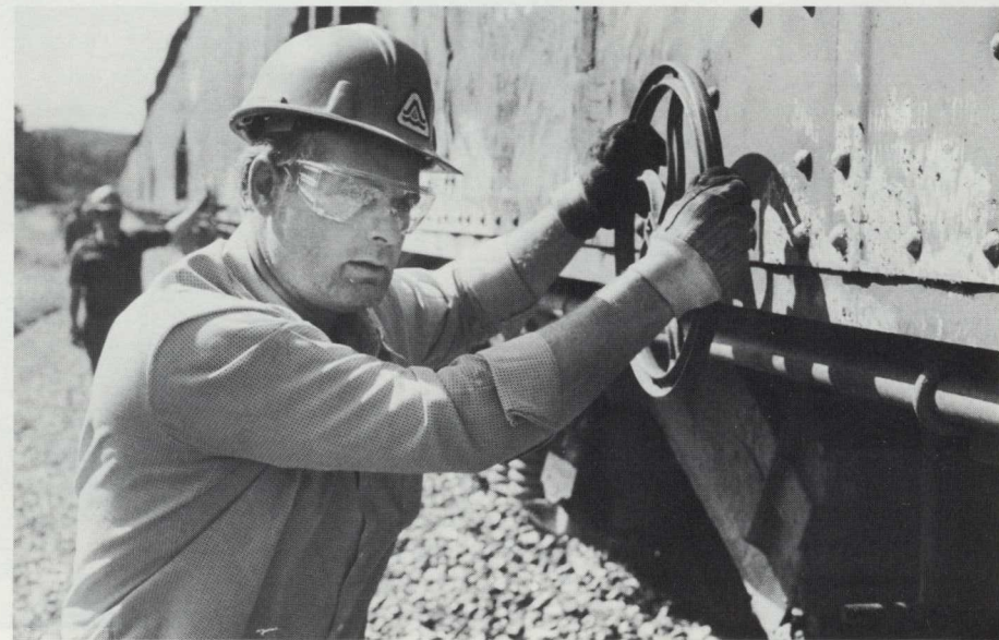
In order to put out the greatly-increased amount of ballast the regular Ballast Crew had to borrow labor from local Section Crews. Trackman Delman Pelletier, Fort Kent, was working just north of Portage when this photograph was made.
