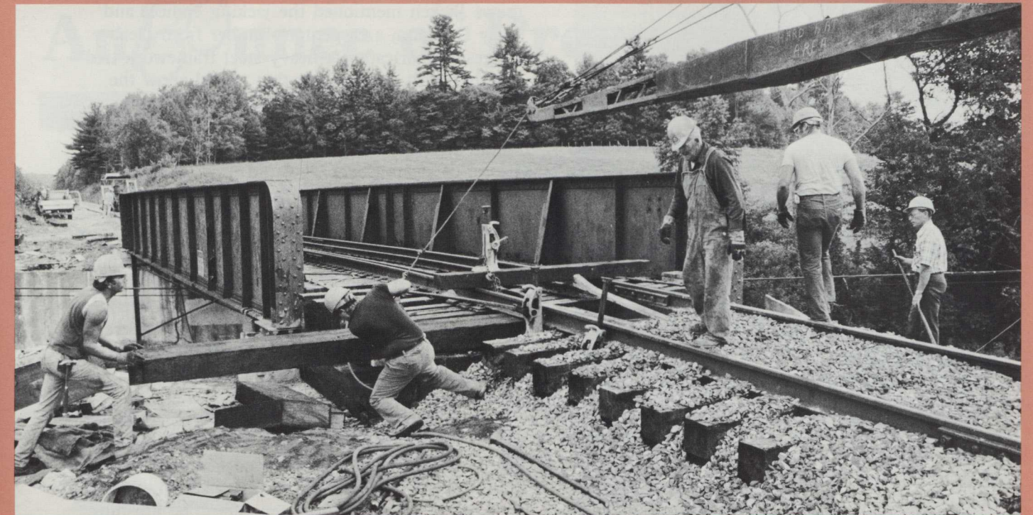
Foreman Eddie Burton, pictured at center, and his crew raised the 60 foot, 124,000 ton bridge in six weeks. The job was made easier with Gary Dunham's "better mousetrap".
