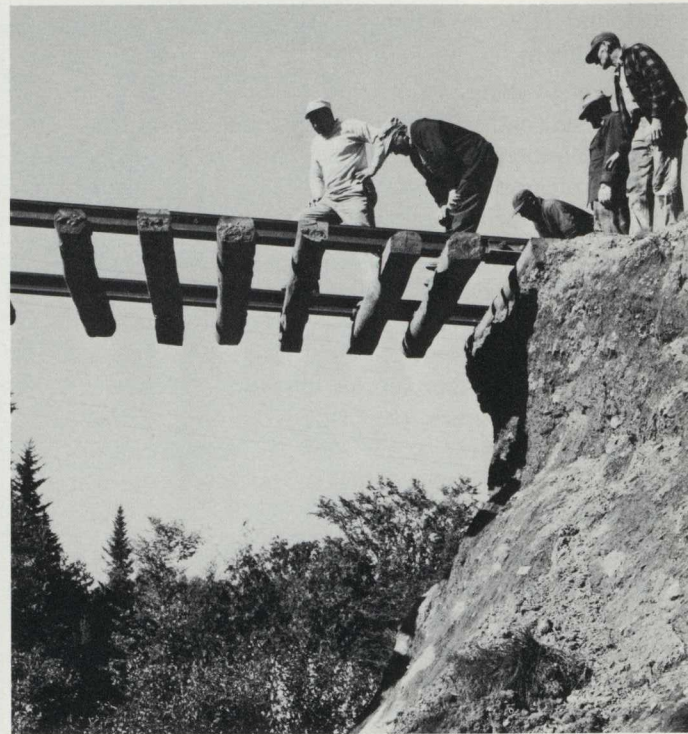
Sagging and unsupported ties and steel were common sights throughout Bangor and Aroostook's system. Train service was virtually non-existent the first 48 hours after the storm. Track forces were quickly mobilized and work begun on the 157 washouts caused by the storm. People who remember it say that more gravel was taken from Horseback Pit at Houlton during the first 24 hours after the storm than normally would have been used in a week of heavy summer use.
