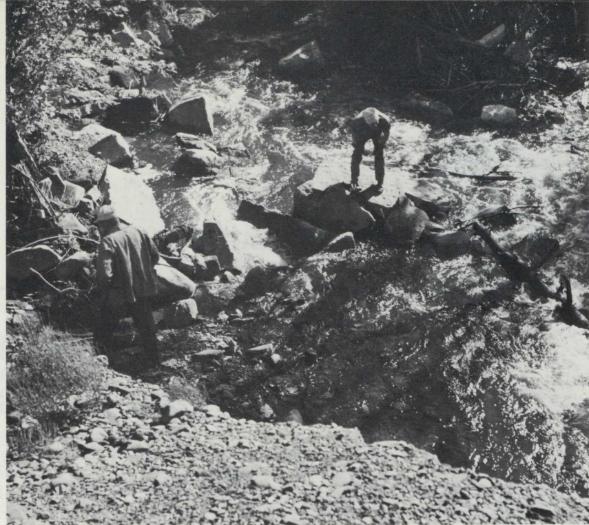
Two track workers examine massive pieces of granite washed out from a culvert on main line track.
