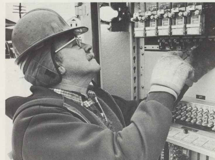
Signalman Bob Pratt works alongside of factory representatives installing the new electronic signal system at Millinocket.
