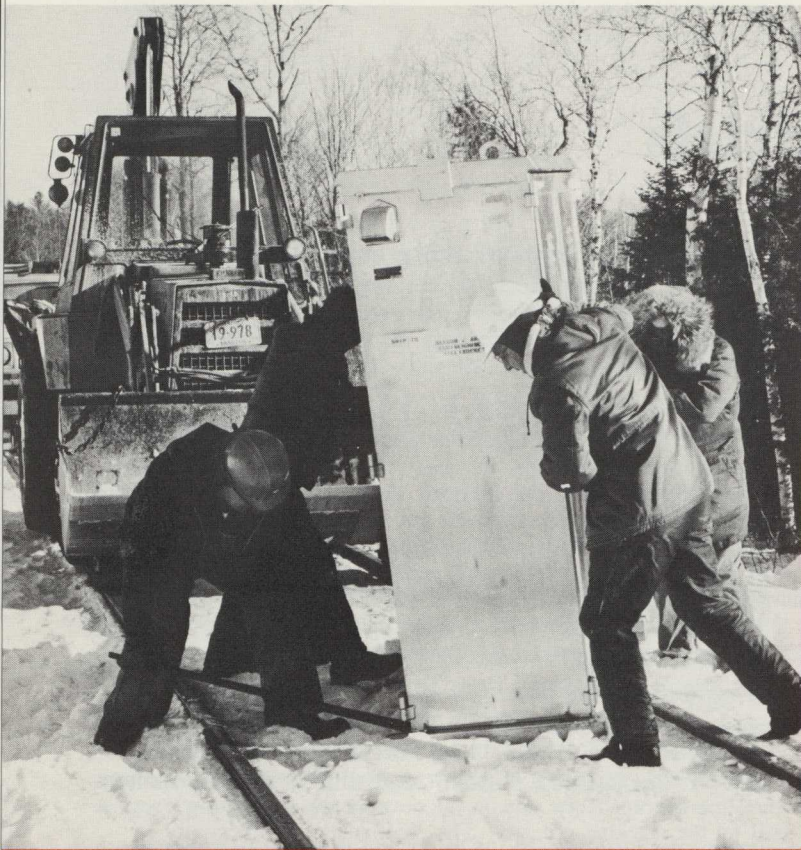
Using a high-rail equipped tractor with a frontend loader, a small signals crew installs a new case with electronic components as part of the new signals system in Millinocket. In 1958 while maintaining its own telegraph system and telephone lines, BAR employed a peak of 26 people in its signals and communications effort. The number has shrunk to five due to changes in technology and work requirements.
