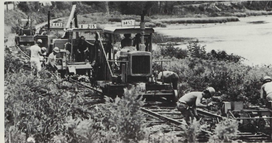
The many branch lines on American railroads are falling into disuse and being abandoned, but Bangor and Aroostook's Limestone Branch has escaped that fate, due largely to the needs of Loring Air Force Base located at the end of the branch. Machines of the tie crew are concentrated in this photograph on the banks of the Aroostook River outside of Caribou.
