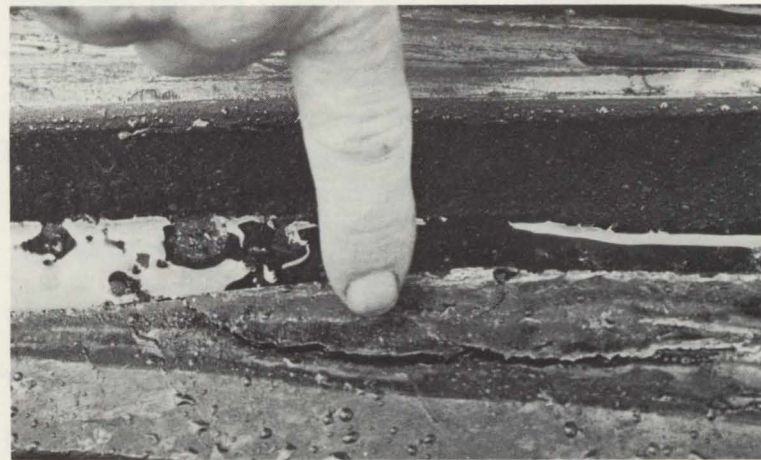
Switch points and points of frogs are vulnerable to wear and batter from steel wheels as indicated in this photograph of a frog point. It's one of the defects that Cole must watch for in his daily patrols.
