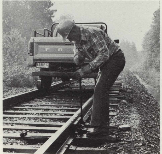
Loose nuts and bolts are frequent defects and Cole is in and out of his truck dozens of times a day to tighten them. But it takes sharp eyes to spot these from a moving vehicle.
