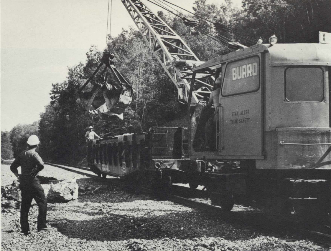
A Burro crane unloads riprap which is being installed on the side of track along the St. John River.
