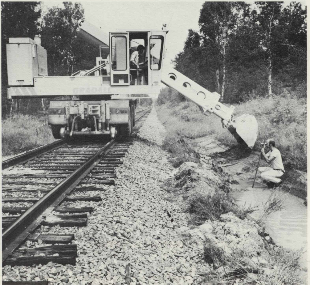
Jeff Lawlor takes a sighting on the track to determine the proper depth of the ditch, while Andrew St. Amant operates the controls of the Gradall.
