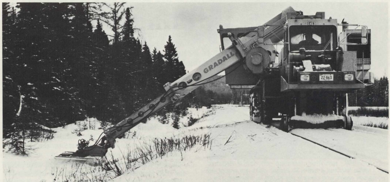
After the ditching season is over and the ground is frozen, the Gradall unit becomes a brush cutting machine, pictured above, and can handle about four miles a day until the snow becomes so deep that brush cutting is not practical.
