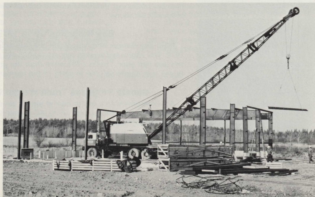
A crew from AGI, the contracting firm that built the new garage, began erection of the steel-work last fall. The building was designed with energy conservation as a major consideration and is heavily insulated. The railroad's 28 motor vehicles in the area will also be serviced at the garage.
