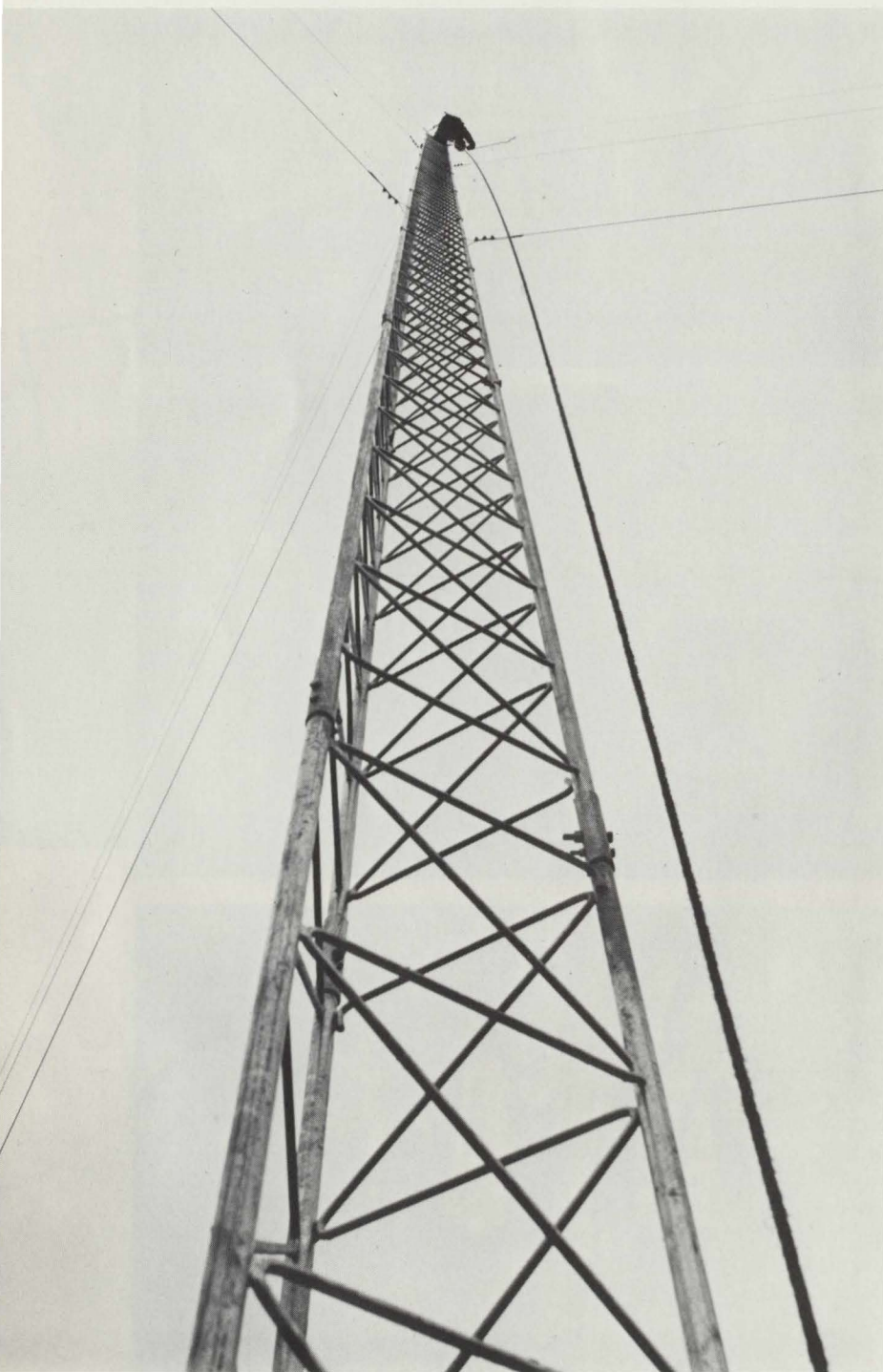
The speck atop the railroad's new 100-foot antenna tower on Parkhurst mountain in Presque Isle is Bob McPhereson, of Aroostook Communications, Inc., the Motorola representative who erected the tower and installed the antenna. The new facilities will house a repeater system that will broaden the road's radio capabilities and provide a more versatile system. Completion of the new radio system will replace all telephone communications on the Northern Division with radio.
