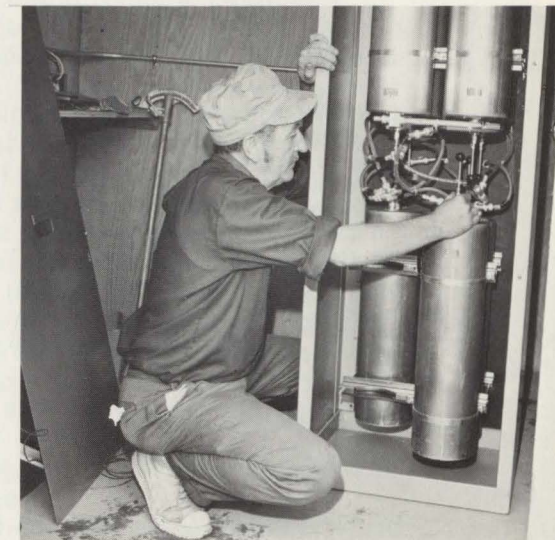
Radio Maintainer Darwin Turner works on a cabinet containing $1200 worth of cavity filters, electronic devices that separate the company's assigned radio frequencies.
