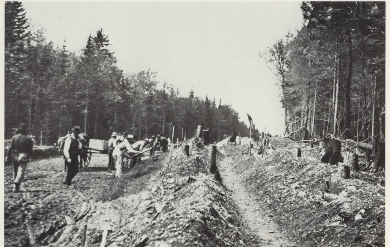
This grading crew was working near Portage during the construction of the Fish River Railroad (later to become the BAR's Ashland Branch) when this photograph was made just after the turn of the century. The last tree that was felled to build the BAR struck the earth 62 years ago. The tree most recently felled to build highways in northern Maine came down today.
