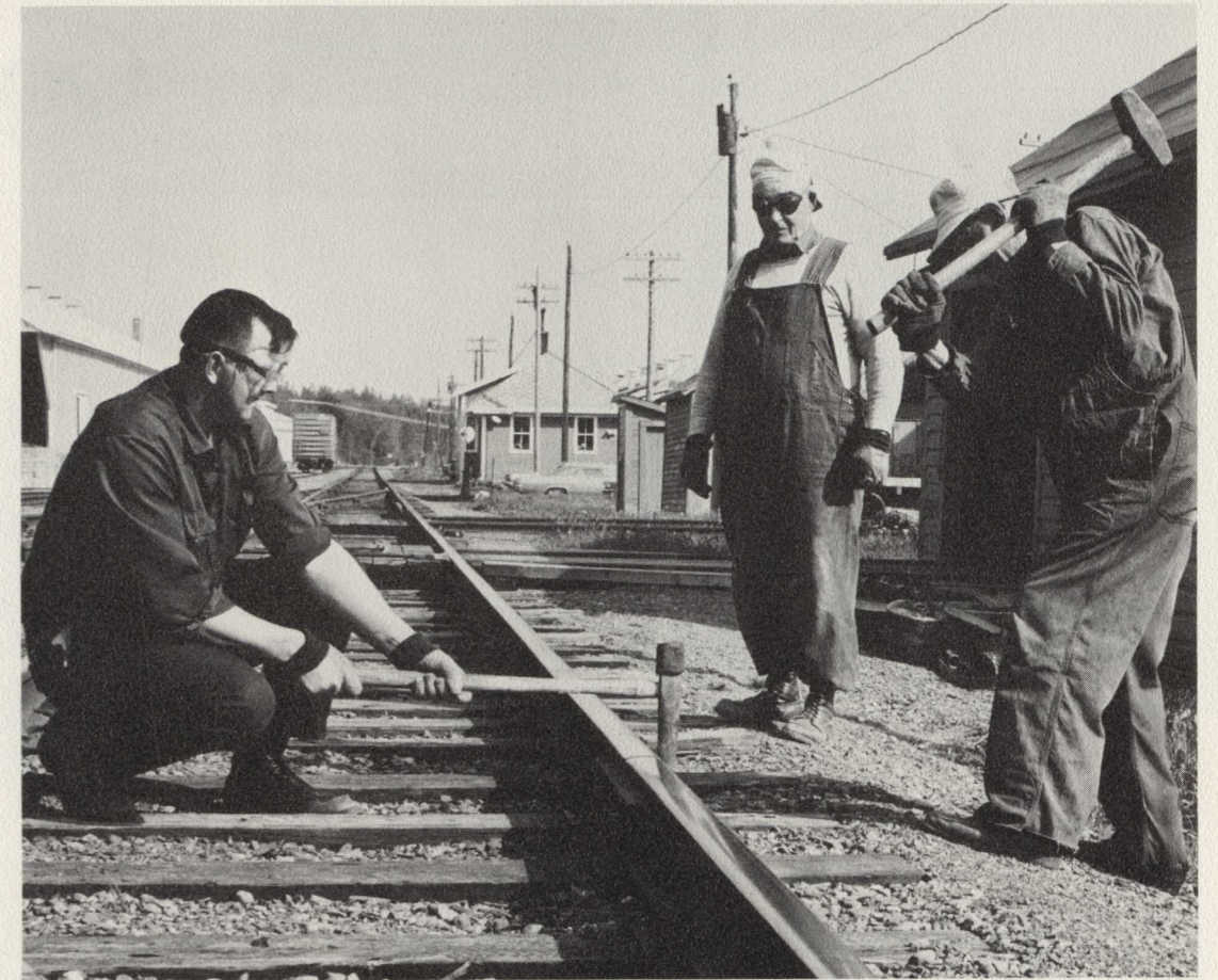
Danger from flying bits of steel is a hazard when Ray Foster's crew cuts a track bolt with a chisel and every man wears protective goggles. The chisel, held by Trackman Harold Ewings, is padded with rubber to minimize the possibility of bits of steel breaking off when Trackman L. D. Sweenor strikes it with his hammer.
