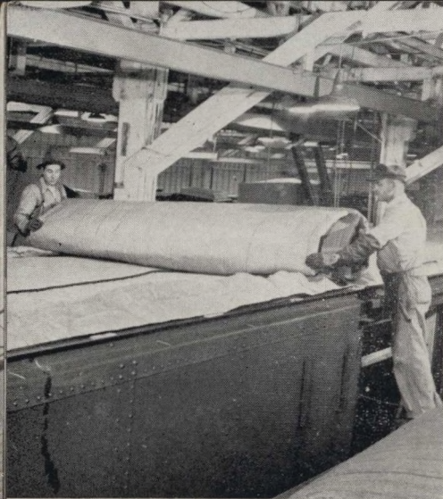
Insulation is added to roof frame before final roofing is put on.
